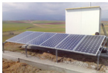
Solar Photovoltaik Telekommunikationssystem Solar photovoltaic telecom system
